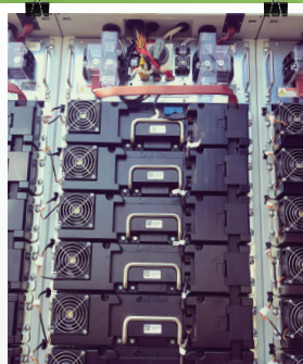
KEARNY MESA BATTERY STORAGE PROJECT
